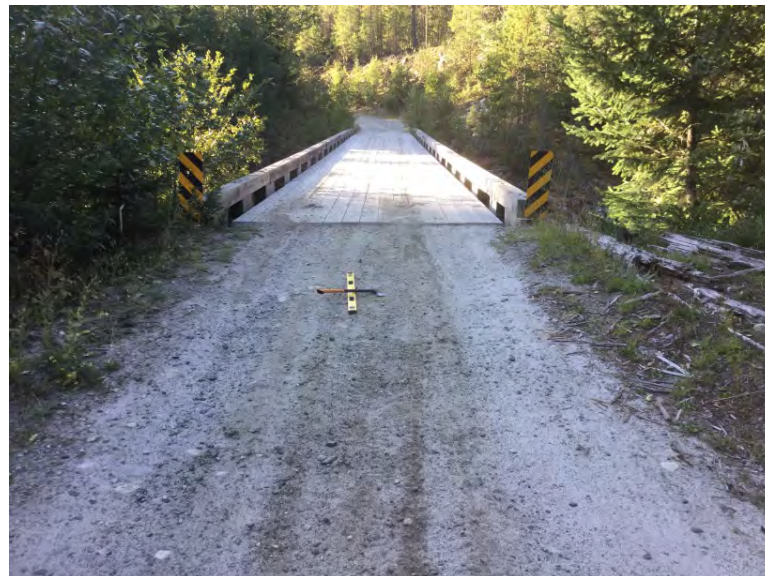
Fender logs rotten or missing at left bank
