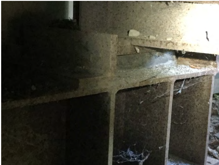
Upstream right bank bearing, rubber bearing pad deformation
