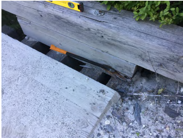
Some risers in poor condition and all hardware loose
