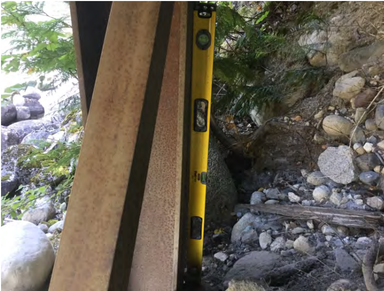
Downstream Pier pile is leaning slightly towards right bank (into fill)
