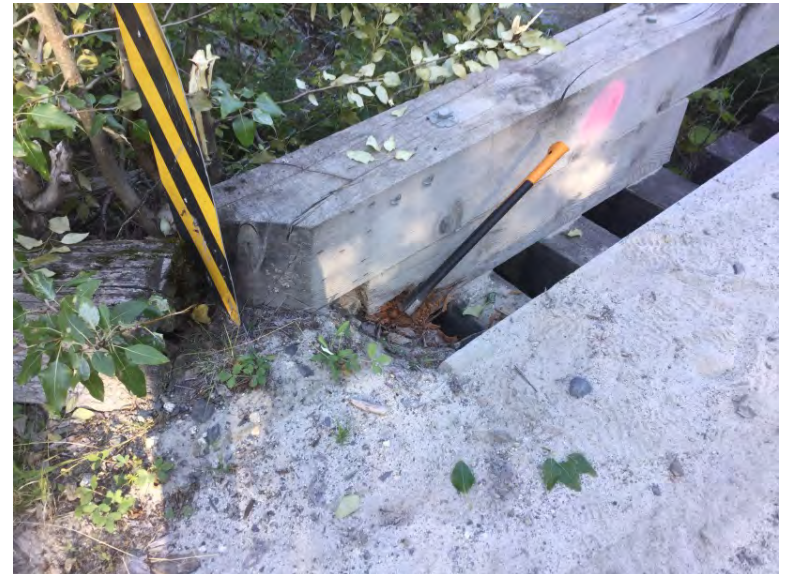
Rotten risers and hardware loose
