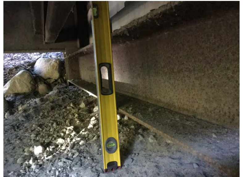
Right bank cap leaning towards stream
